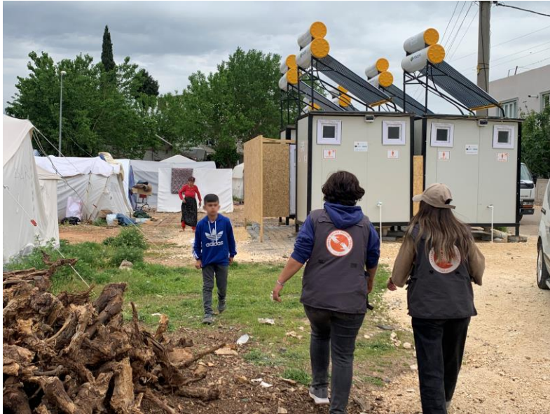
3. Installation of a water tank with solar panels to meet the hot water needs of toilets and showers, Adiyaman
