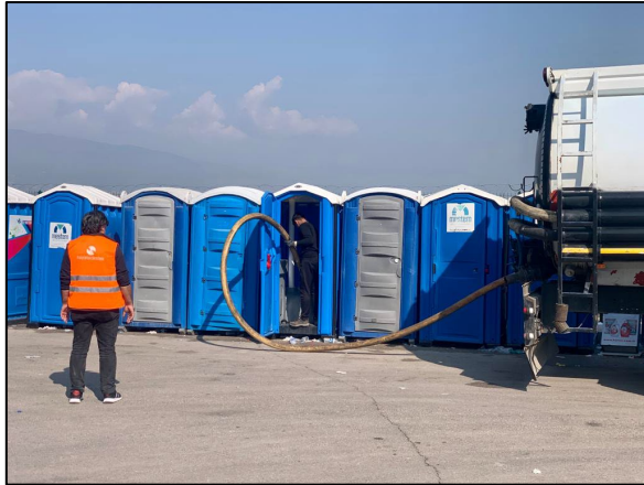
2 Portable latrines located in Hatay
