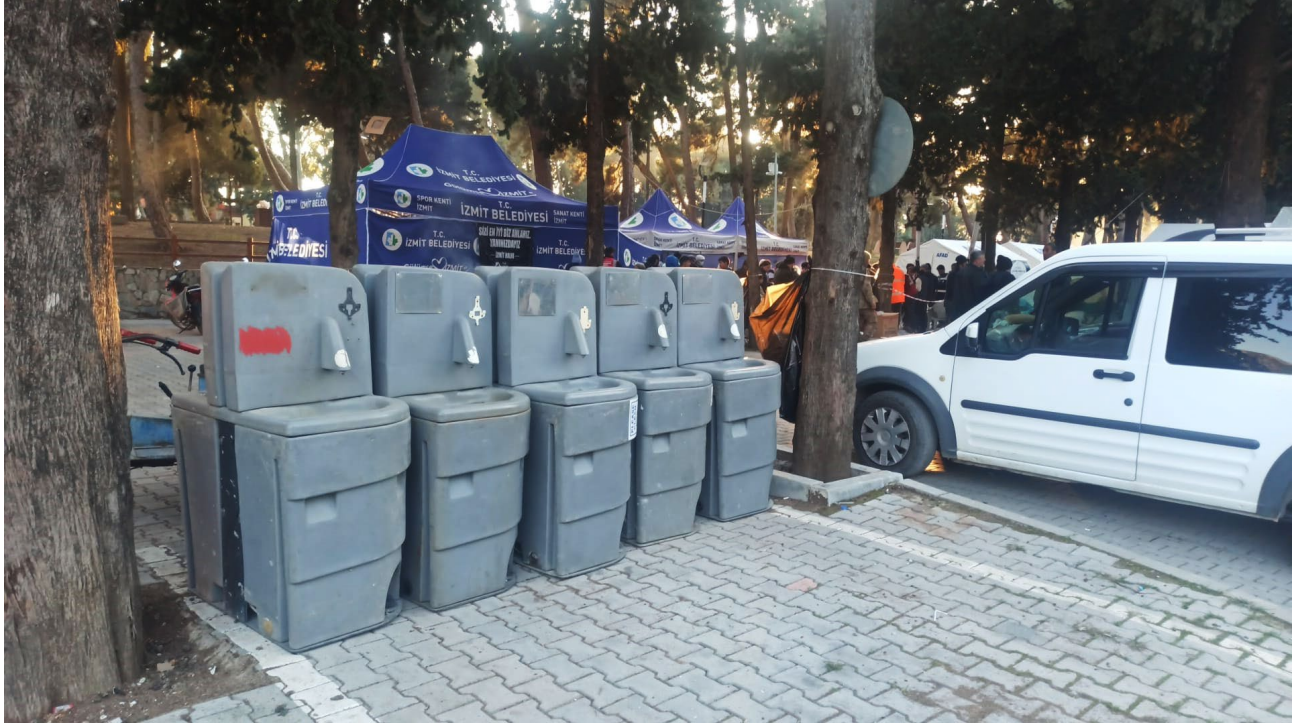
Handwashing units are installed in multiple points in Defne. STL WASH program is being rolled out across the affected region.
